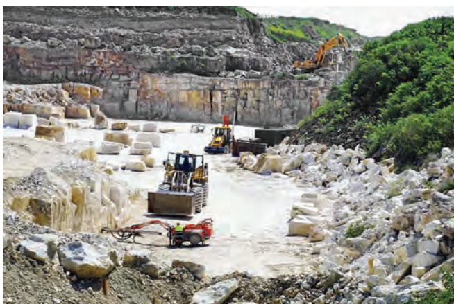
Broadcroft Opencast Quarry looking southeast. A drilling machine placing holes for blasting – the front loader appears to be carrying a steel box, perhaps containing the black powder charges. A mobile saw in the background with cut blocks drying. Harder overburden over desirable stone can be seen in quarry face
